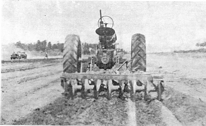
◀ Soil stabilisation in progress. Gobble disc harrow mixing 'kabook', sand and water to form a base
